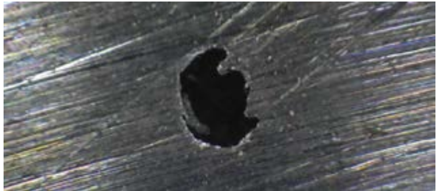
Example of a corrosion pit. Visual inspection of the pit provides no information about the damage to the subsurface
