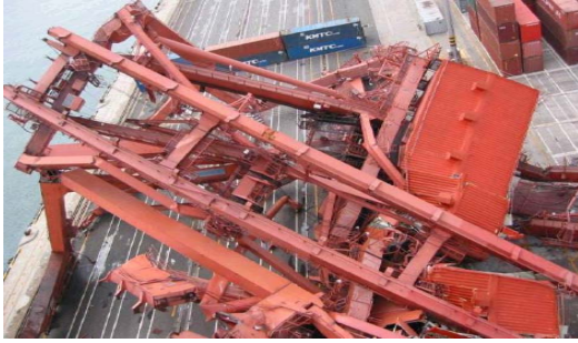
PICTURE: WINDSTORM DAMAGE
