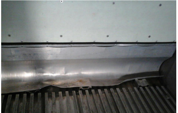
Picture 13 Damage to machinery airflow baffle.
