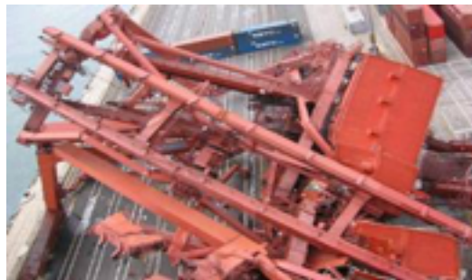
Figures 5 & 6: Examples of wind damage
